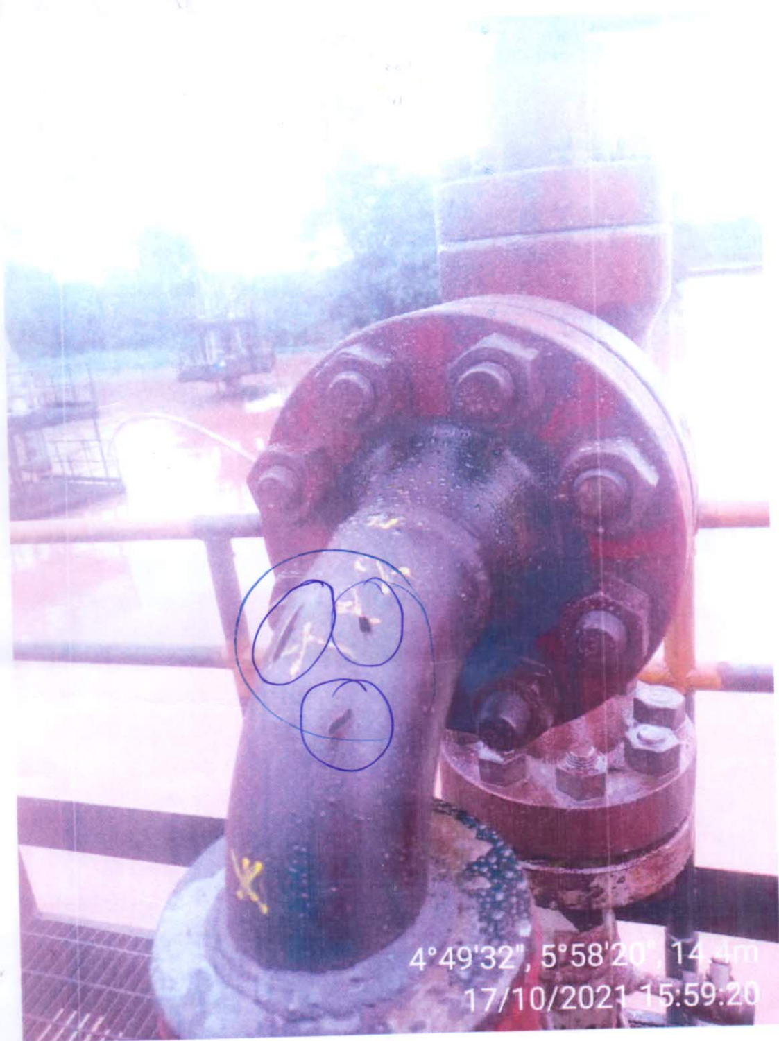
SPILL POINT ON THE WELL HEAD
